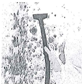
Black Mold Removal
