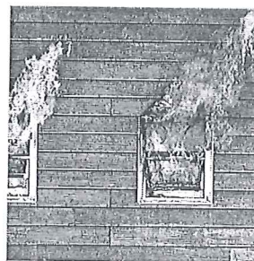
Fire and Smoke Damage
